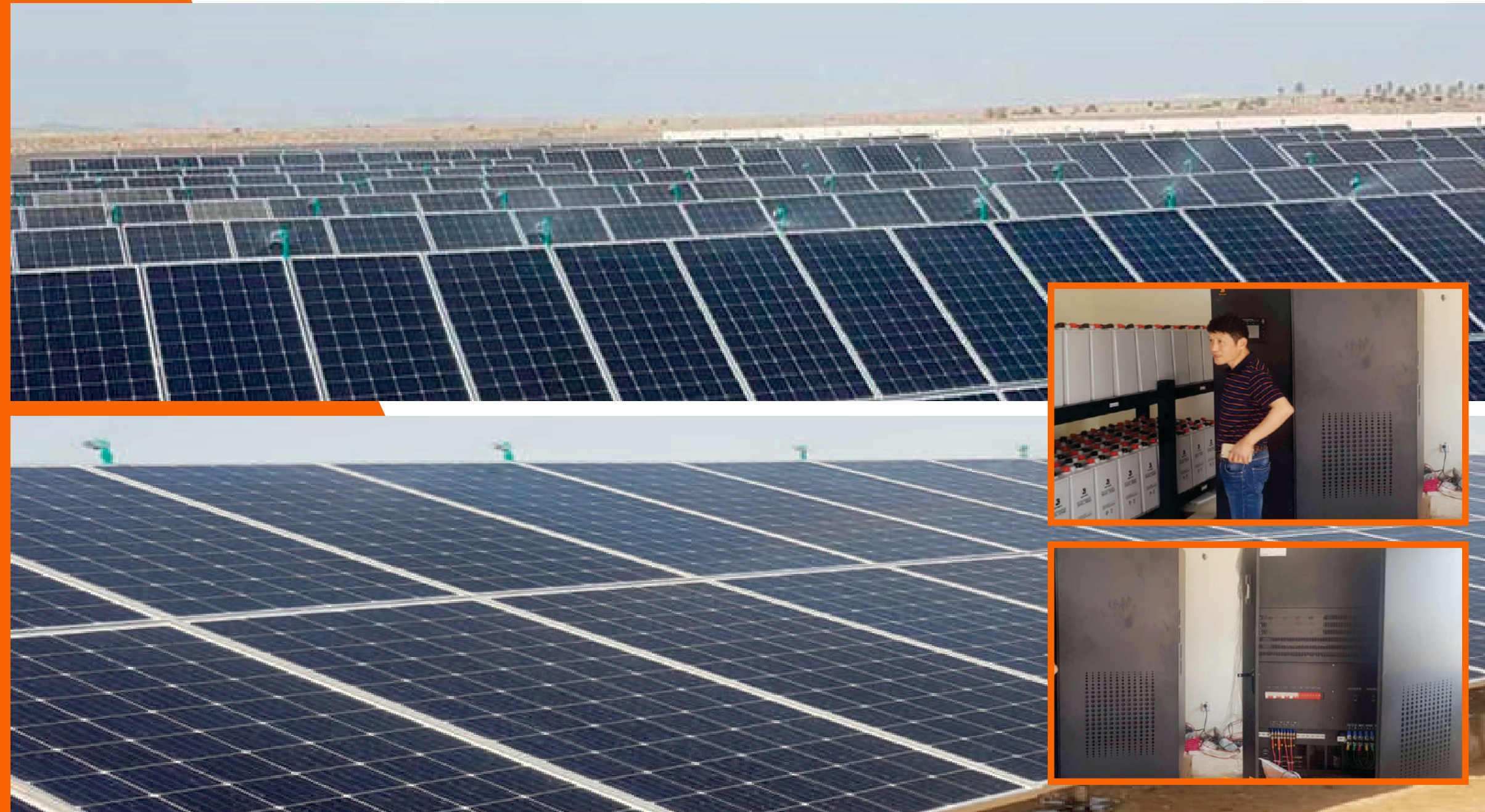
ORMARA 160kW SOLAR PROJECT
