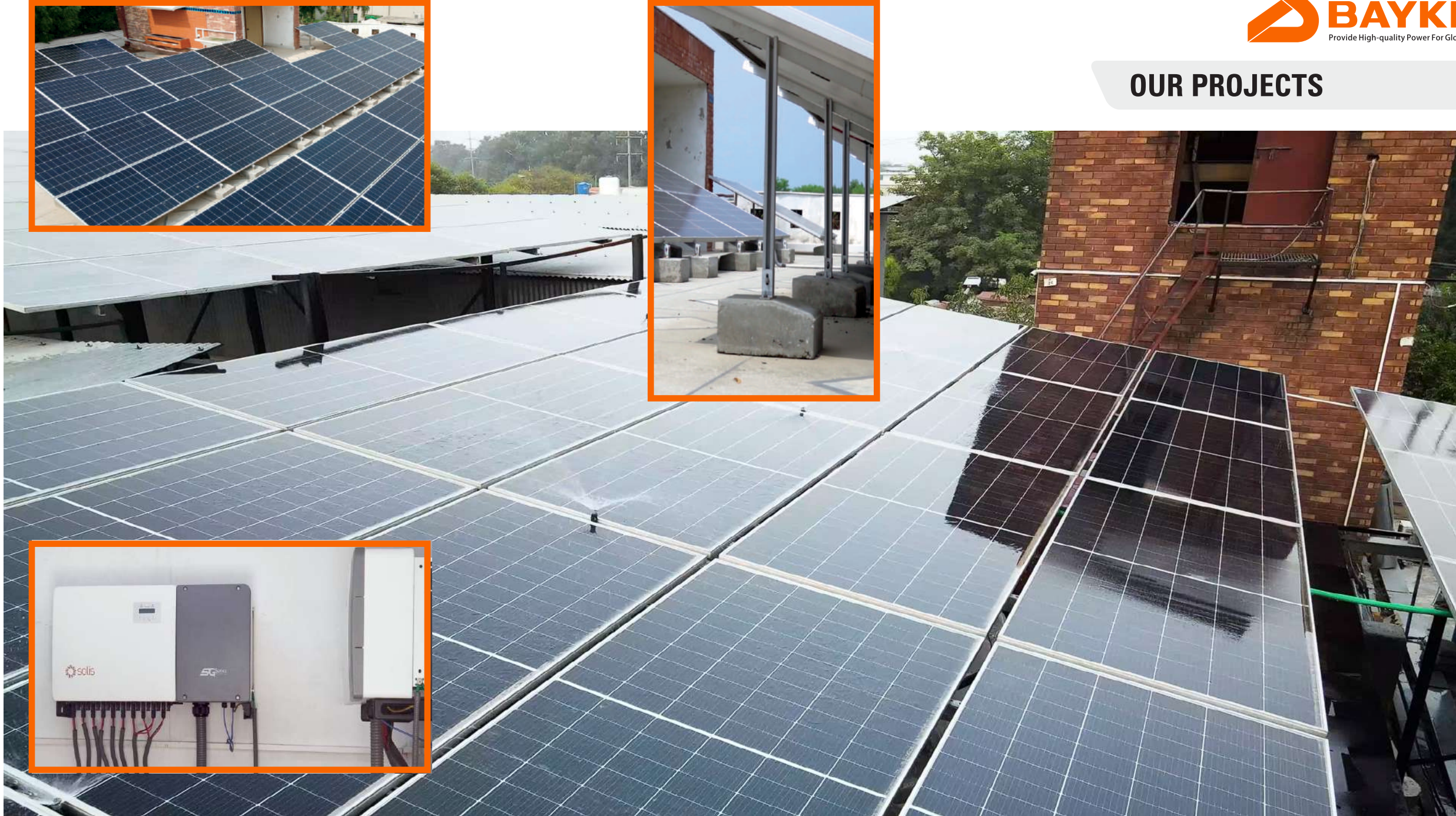
450 Kw SOLAR SYSTEM IN LAHORE
